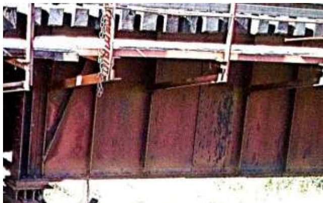
5.21-rasm. Mahalliy korroziya
