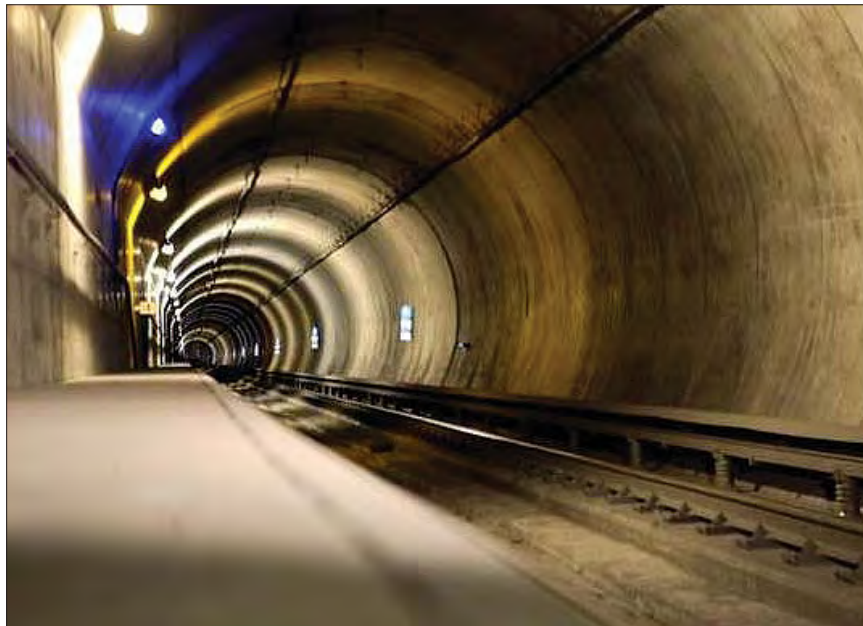
The BART network runs more than 30 miles through subways and tunnels such as the Transbay Tube.
